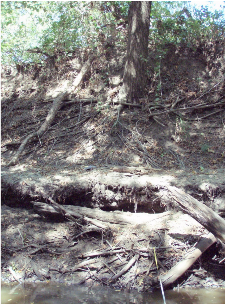
Figure 2. The right bank at station 18770 on Tehuacana Creek, September 2006.
