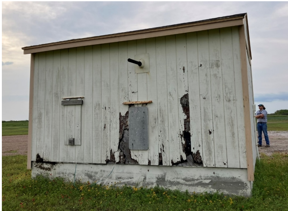
4. Generator shed: Bee colony in wall will be removed by TPWD before roofing. Wall panels not in contract.
