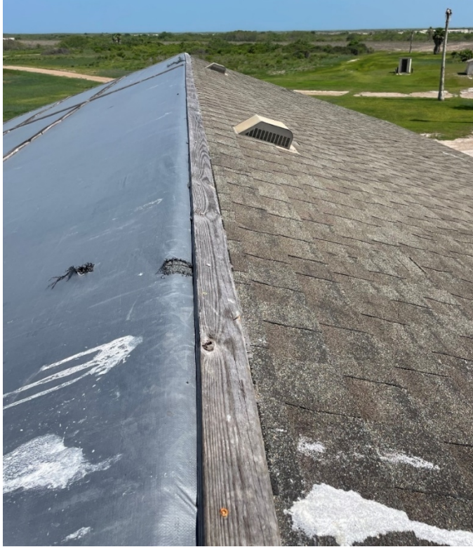
3. Garage roof; roof vents along ridge. The black tarping on the damaged area is deteriorating.
