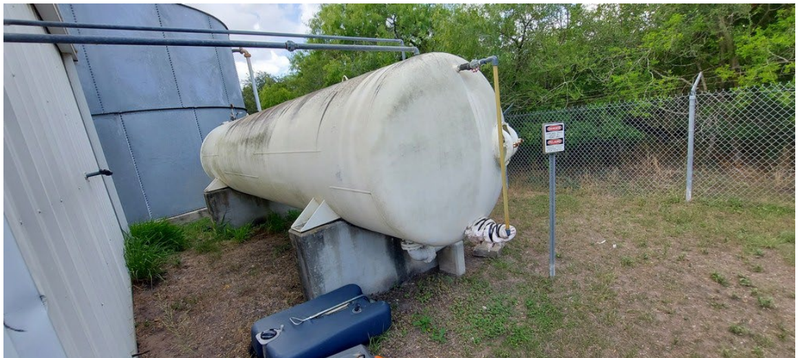
Existing Hydropneumatic Tank. New Air Charging Compressor shall be installed on tank
