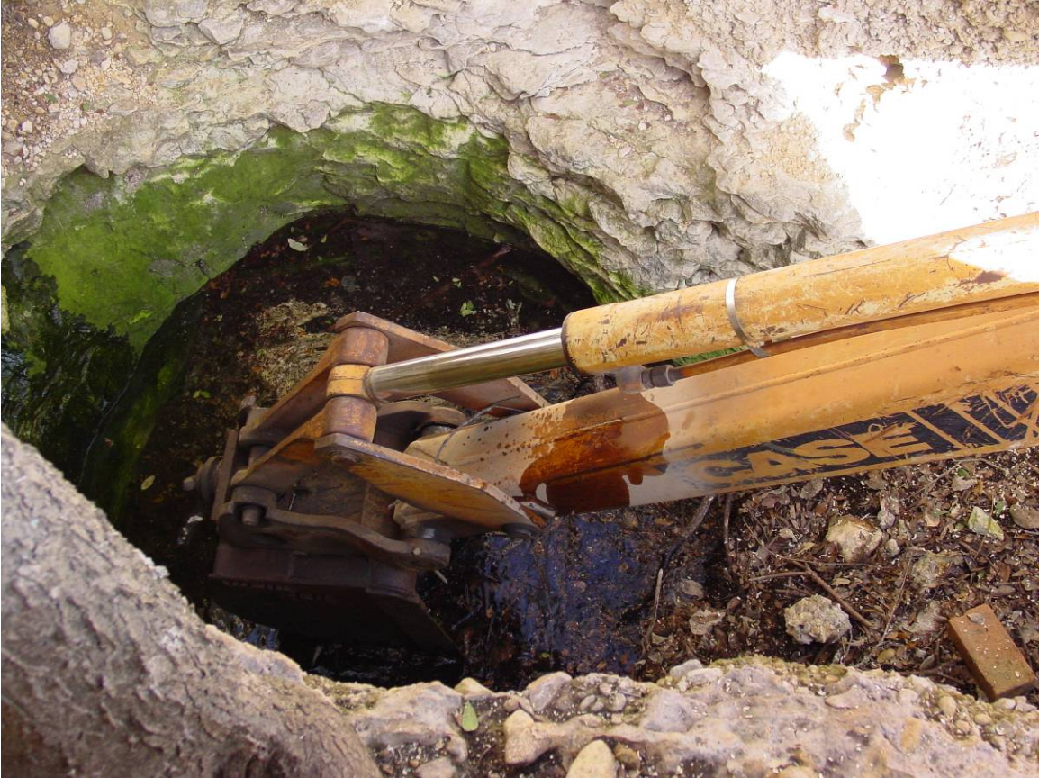
Figure 4. Excavation of Dowell Spring using a backhoe. The backhoe encountered a solid bedrock bottom approximately 0.75 m below the surface of the water.
