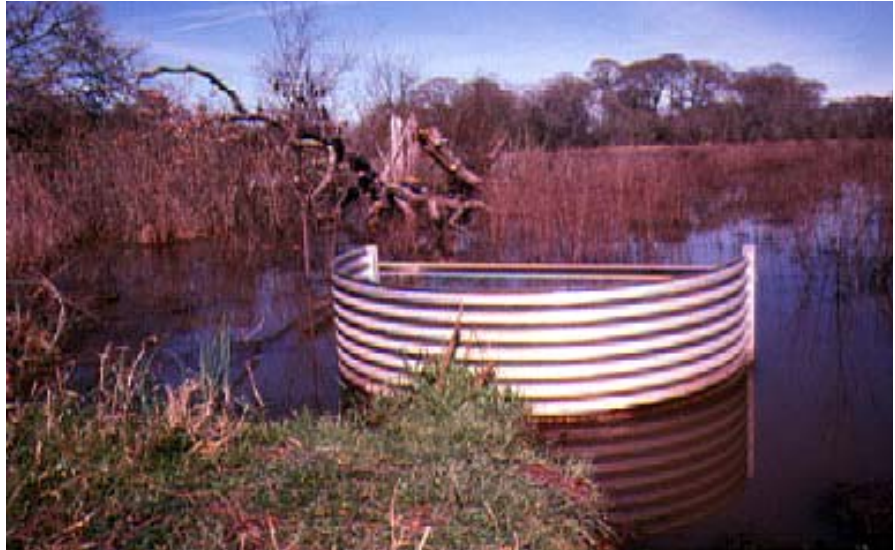
A flashboard riser box attaches to a pipe installed in a levee to create a shallow water wetland for wildlife.
