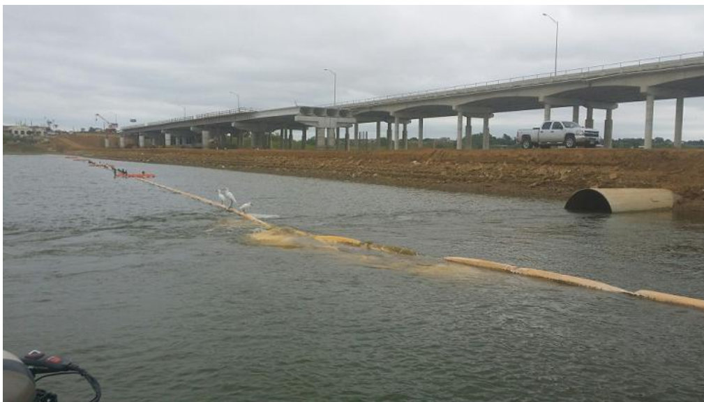
Figure 2. Photos of the earthen construction levee that prevents navigation under the Highway 83 Bridge, April 2016, Falcon Reservoir, Texas.
