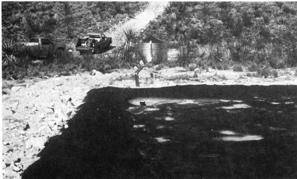
Figure 13 Rainwater catchments can be made out of asphalt impregnated polyester fabric.
