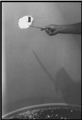
The woodpeckers pecked through the outside wood, then through the sheetrock, and into the house. This hole measured about 5"x6".
