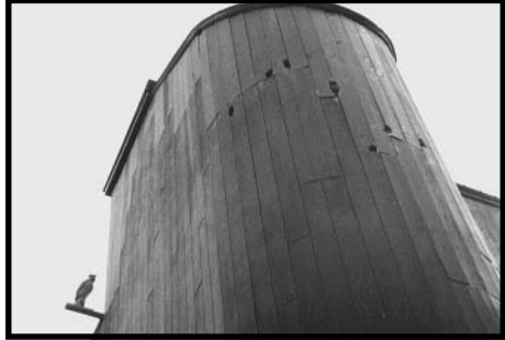
Seven holes are visible here, some with insulation hanging out. These holes measure at least 5"x5" each. Notice the ineffective owl decoy in the lower left-hand corner.
