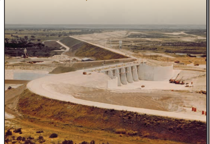
The Choke Canyon Dam under construction, 1982. Photo courtesy U.S. Bureau of Reclamation.
