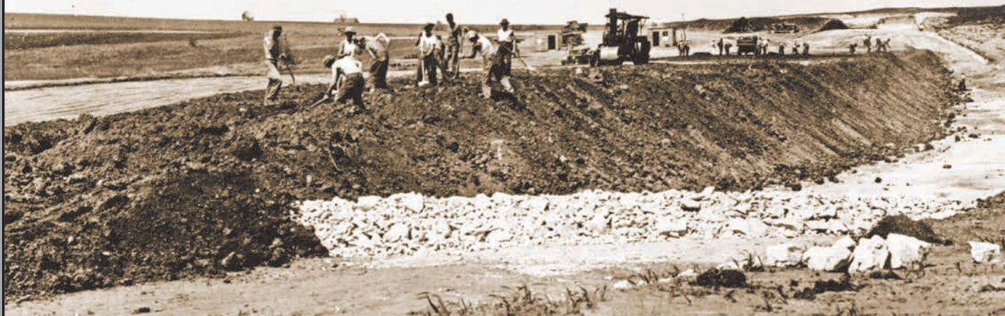
Construction of the Dam, 1934. Using hand tools, enrollees in Company 894 work the sloped side of the earthen dam.
