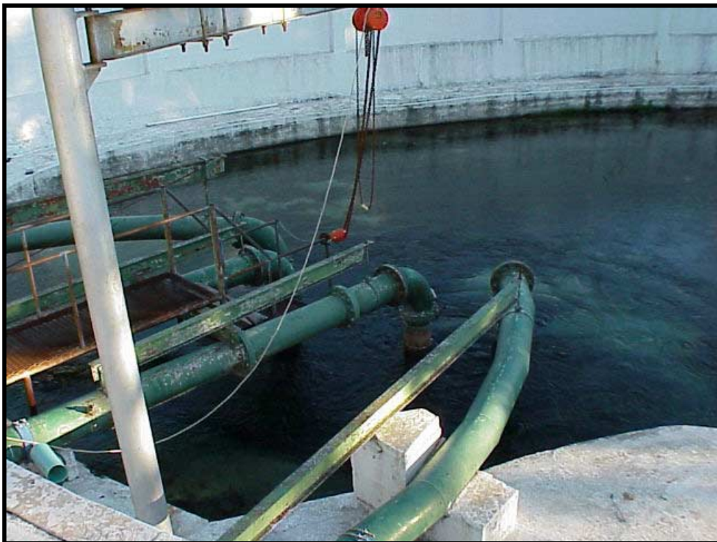
Figure 41. City of Del Rio municipal water intake at one of the springs. This spring produces 90 million gallons a day (11/20/00).
